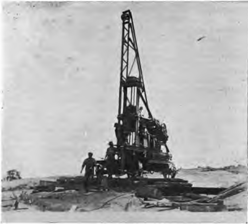
PLATE 184a. —Contract 9. Deep Hole or Traction Drill. Temple-Ingersoll Electric Air Drill Mounted on Front of Machine; Entire Apparatus Motor Driven. Drills holes up to 30 feet in depth for deep cuts in quarry.
